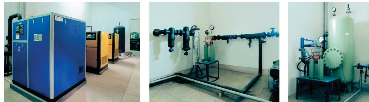
Performance testing room
